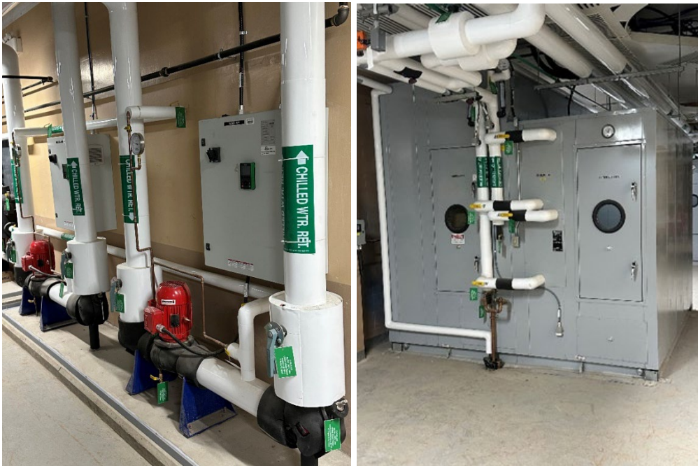
Figure 9a: New chilled water supply piping Figure 9b: One (1) of four (4) new air handling units
