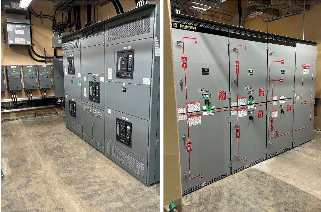
Figure 10a: New 600v switchgear electrical panels Figure 10b: New 4160v switchgear electrical panels
