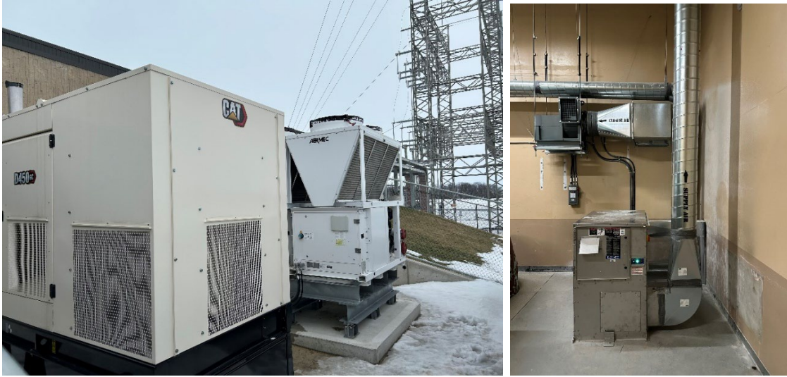
Figure 8a: New diesel generator set, and new chillers Figure 8b: Example of a new dehumidification unit
