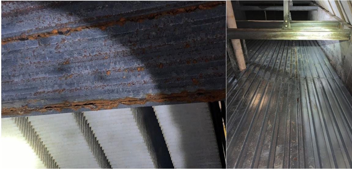
Figure 7a: The old clarifier ramp (view of the underside). Corrosion and holes in the ramp are evident
