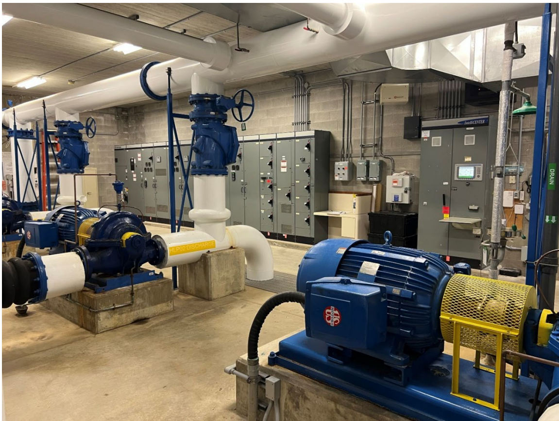
Figure 5: Pump room at the Exeter-Hensall Pump Station (EHPS)
